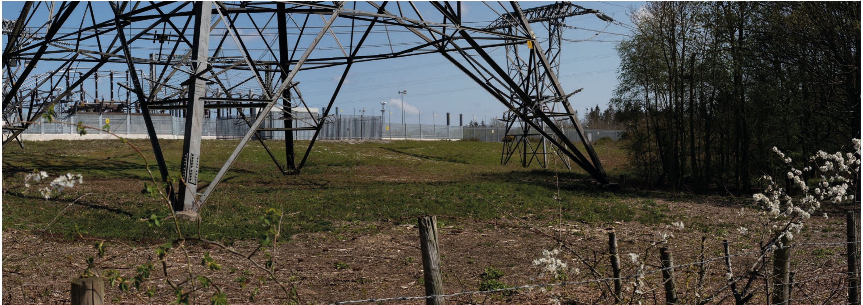
National Grid Norwich Main Substation
